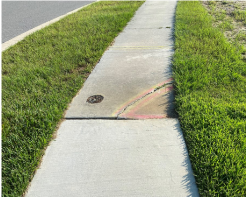
Damaged sidewalk in front of 85475 Fall River Pkwy
