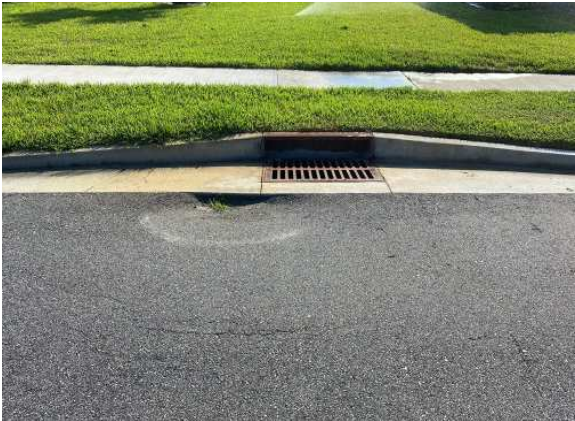
Small pothole near inlet on Fall River Pkwy
