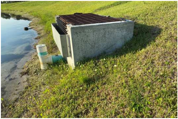
Inlet protection installed on phase 5b pond...also clean out under bottom of orifice pipe
