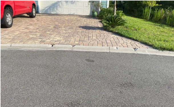
Gutter is chipped in front of 85265 Sagamore Ct
