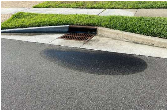
Shallow depression in front of inlet on Fall River Pkwy
