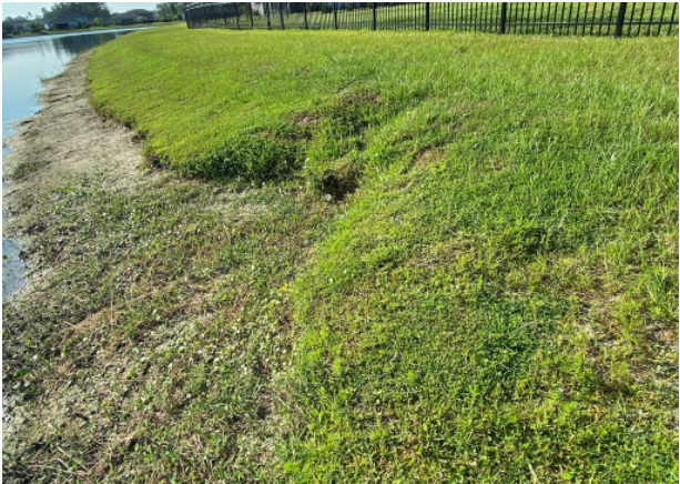
Erosion on phase 4A pond slope
