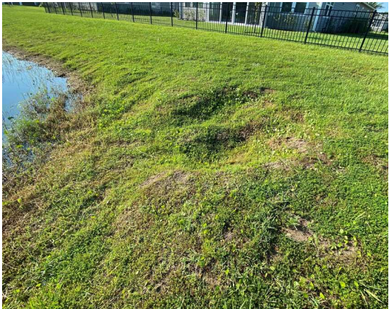
Erosion on phase 4B pond slope
