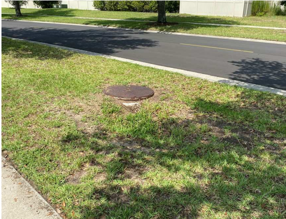
Small hole near storm manhole off Majestic Walk Blvd
