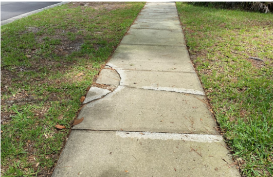
Damaged Sidewalk near roundabout
