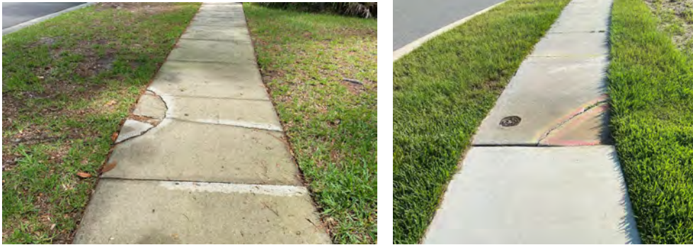
Examples of Damaged Sidewalk
