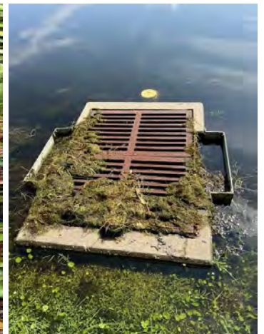
Debris covering Control Structure
