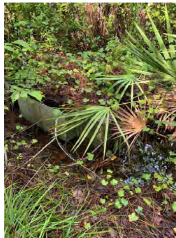
Debris covering Spreader Structure
