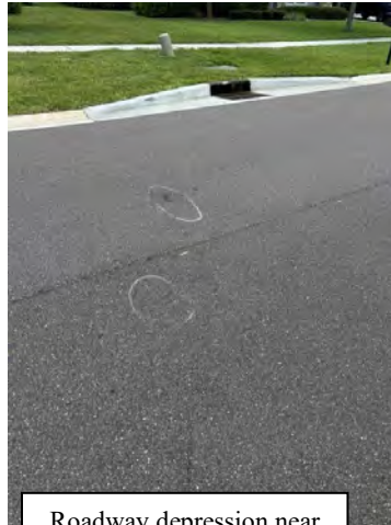
Roadway depression near 85171 MWB
